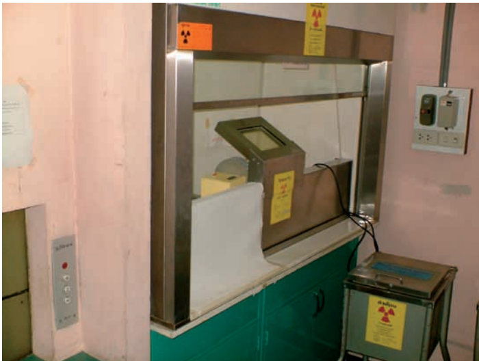
FIG. 5. Typical fume hood.
